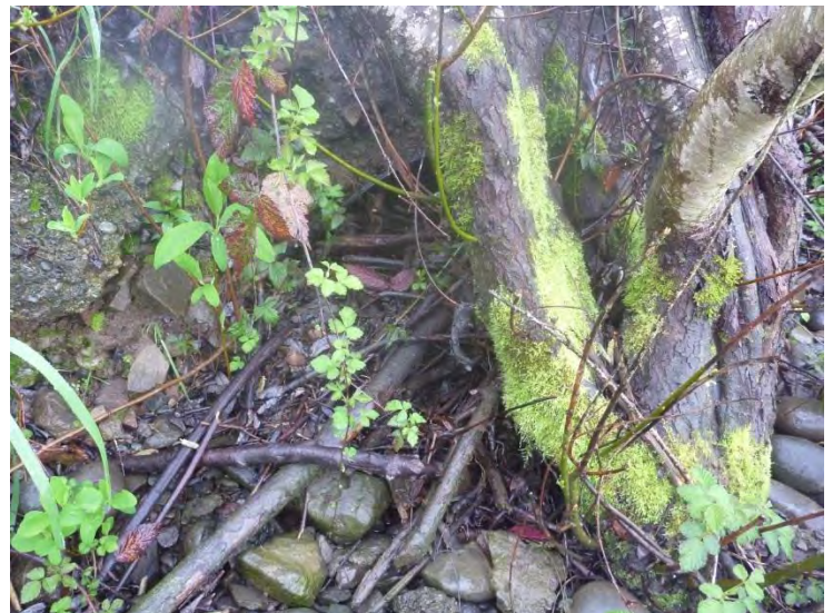
Figure 21. One of the four culverts at Crossing 4 that is plugged with sediment and live growing willows.
