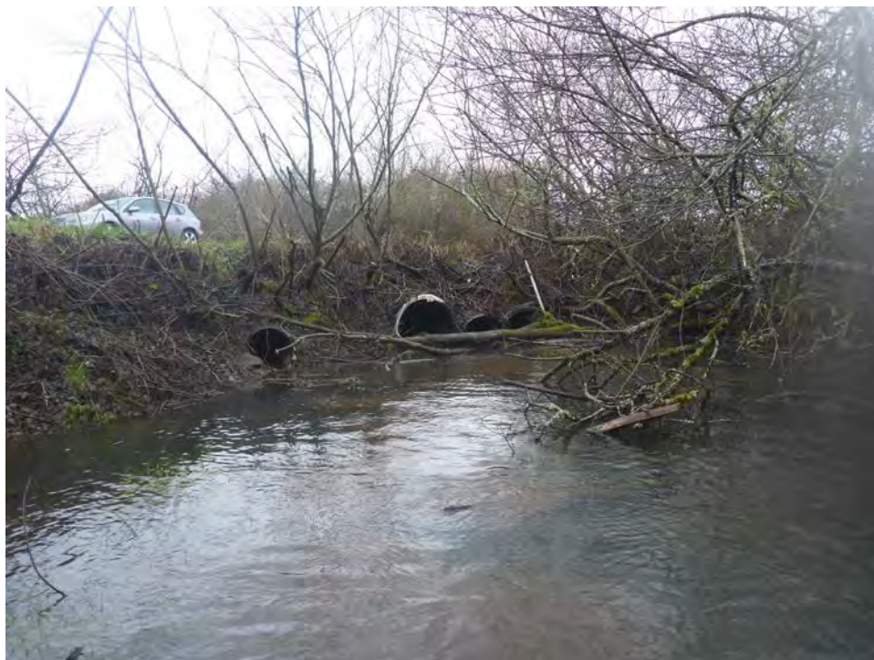
Figure 2-18. Crossing 4 inlet. All four pipe inlets visible. Debris and improper construction cause upstream backwatering. View looking downstream.
