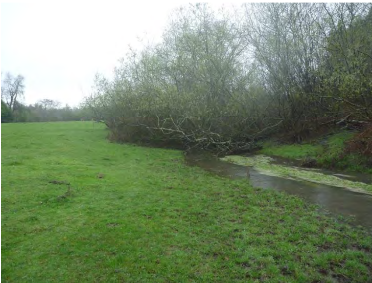
Figure 15. Channel between Crossings 3 and 4 lacks cattle-exclusion fencing. View looking downstream.
