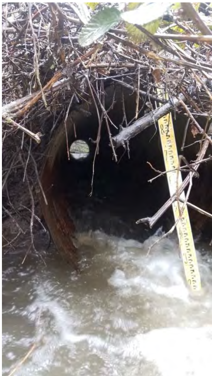
Figure 7. Crossing 1 outlet. Culvert is a 3 ft corrugated metal pipe (CMP) with a shot-gun outlet that is rusting at the base.
