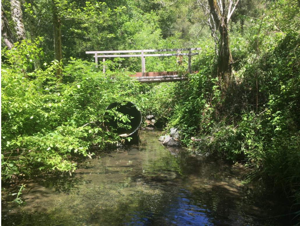
Looking upstream at the project site. Blown out culvert is on the right bank and the weir is on the left bank.
