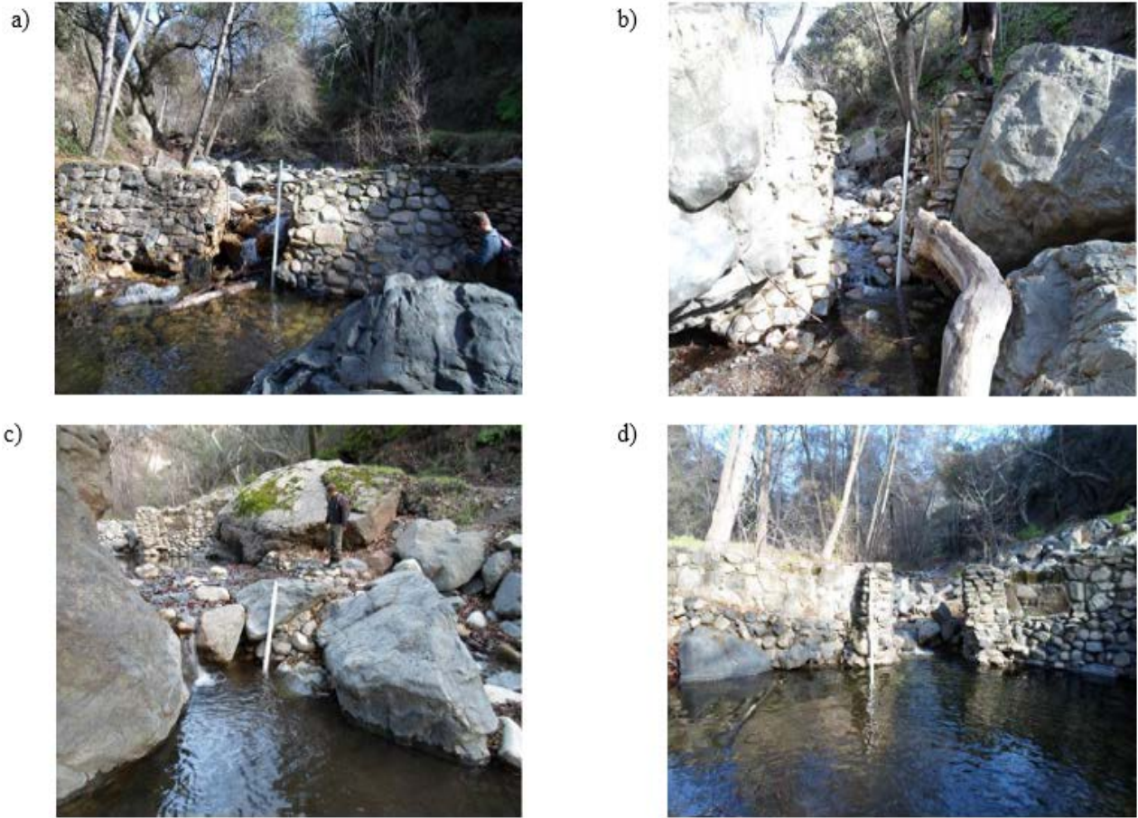
Figure III-3 a-d. Trabuco Creek Fish Dams (TCFD) prior to removal in 2014 a) TCFD7 (6 feet high), b) TCFD9 (4.5-9 feet high at thalweg), c) TCFD10 (2.5 feet high) and d) TCFD11 (6.5 feet high). Photos courtesy of Trabuco Ranger District, Cleveland National Forest.
