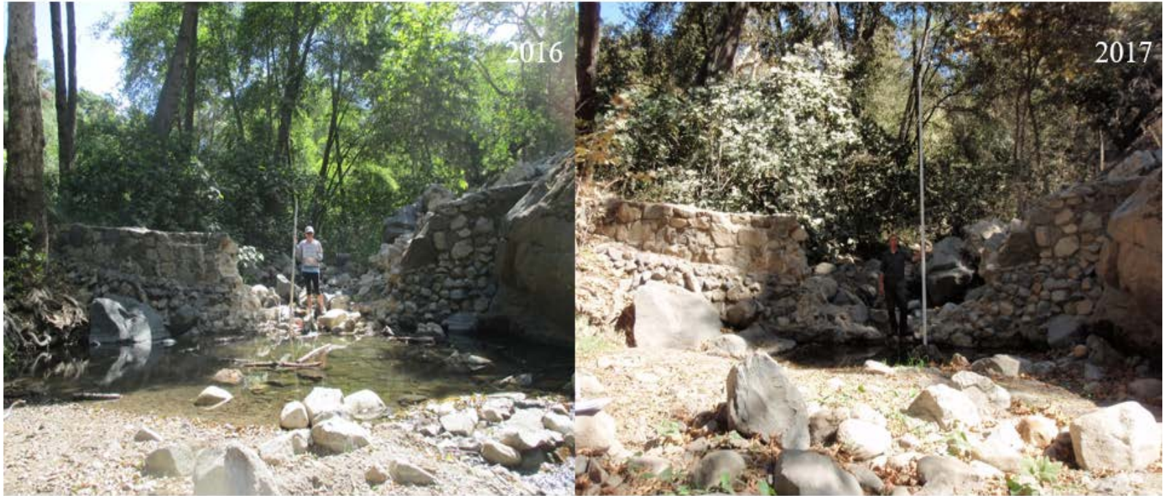
Figure IV-22. Comparison of 2016 vs. 2017 TCFD11 dam removal site . High levels of scour and large boulder movement was observed when conducting monitoring activities in 2017.
