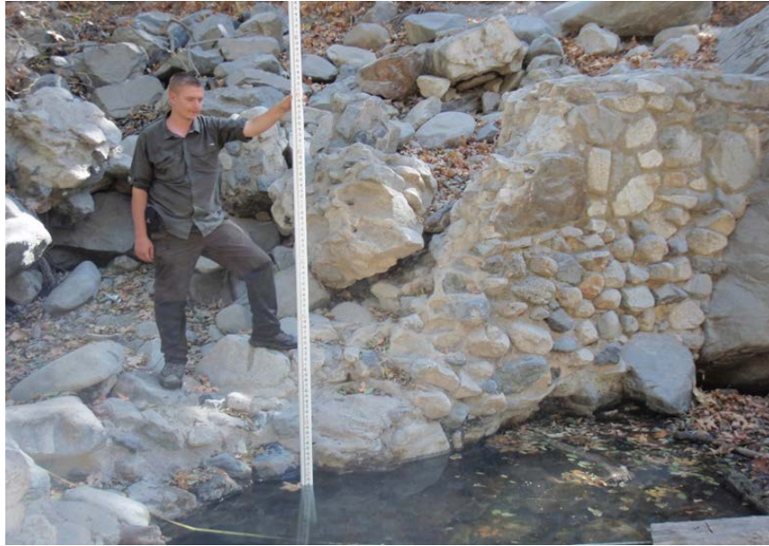
Figure IV-24. TCFD11 in 2017. Significant scour observed in 2017 exposing lower remnant section of TCFD11 creating a small plunge to lower pool with additional scour.
