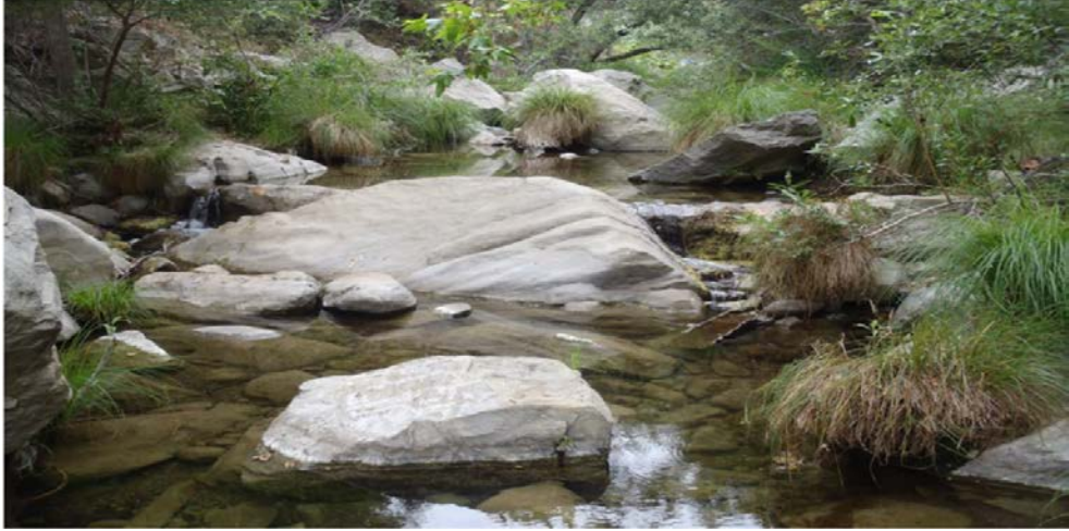
Figure III-2. Arroyo Sequit check dam before removal. Upstream view of small (5 feet high) check dam that was demolished in August-September 2014. Photo courtesy of CCC Camarillo.
