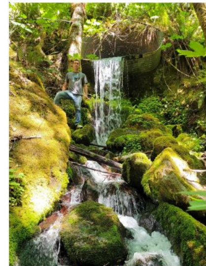
Impassible culvert on a tributary to Knopti Creek, Middle Fork Smith River
