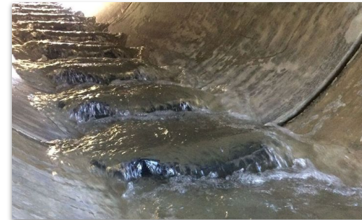
Culvert baffles https://www.ats-environmental.com/
